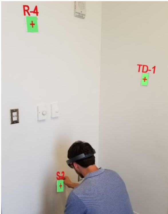
Figure 2: Participant laying out electrical devices with the virtual points shown on the walls around him
