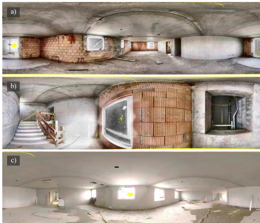
Figure 2: Spherical Point Cloud Renderings of three rooms from the custom validation dataset, collected at a residential apartment building site during shell construction. a) Medium-sized room before plastering work is completed. b) Staircase before plastering work is completed. c) Medium-sized room after plastering work is completed. The scenes are characterized by varying surface textures due to the nature of the construction, challenging lighting conditions, and complex floor plans. They include obstacles and wet spots on the floor, which produce reflections and scanning artifacts. Yellow pixels represent empty canvas pixels where no points were projected.
